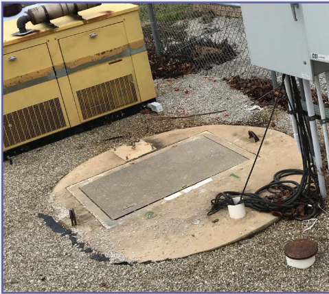
Areas Around Lift Stations
