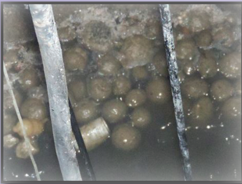
GREASE BALLS & HEAVY ACCUMULATION OF FOG
