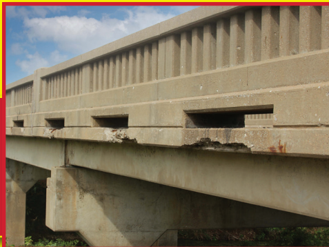
CORRODING DECK DRAINS
