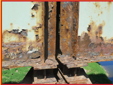
RUSTING BEAM ENDS
