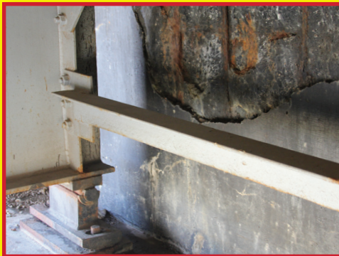
DETERIORATING BACK AND WING WALLS
