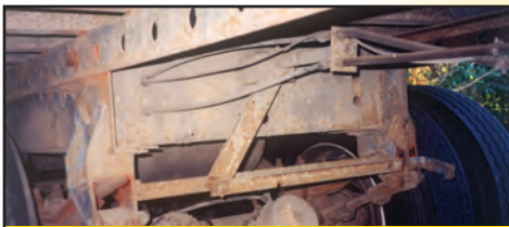
A typical rust damaged frame.
